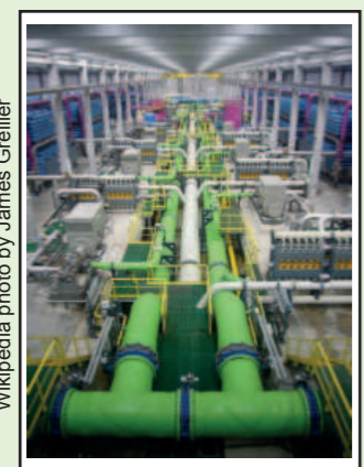
Desalination plant in Barcelona, Spain.
