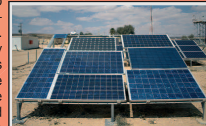
These solar cells in the Israeli desert convert the sun's energy into electricity. (Wikipedia photo by David Shankbone)
